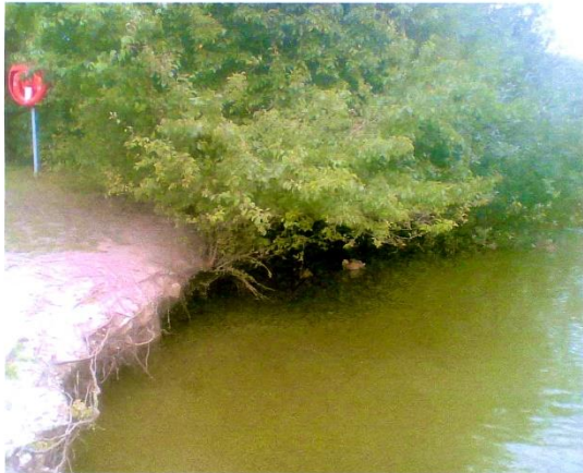
Fig 2. East bank looking south. The bank is badly eroded & is being undercut making it potential dangerous. Reinstatement work will stop at the trees, the branches of which enter the water providing a valuable habitat.
