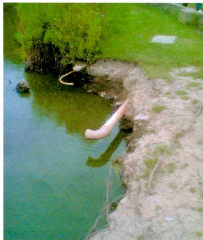
Fig 3 East bank looking north. The overflow pipe shows the level of erosion. This is the main point of public access to the waterside. The pipe feeds into a drain which discharges into a ditch on the Pevensey marshes
